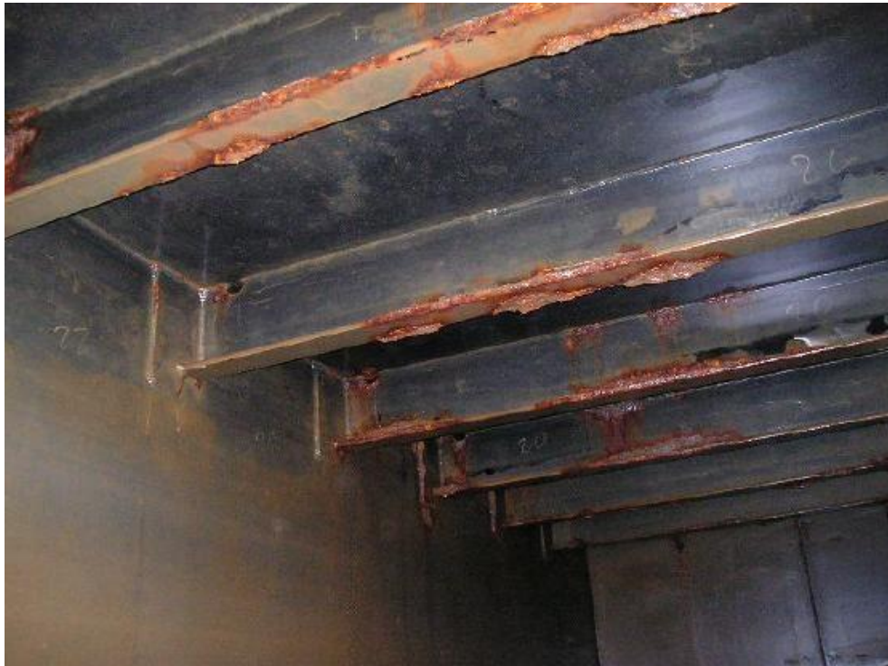
Coating condition changing from GOOD to FAIR but still remaining in GOOD
