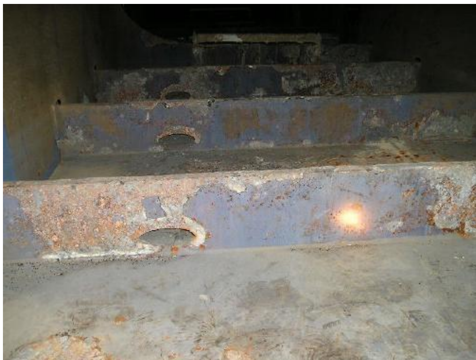
Coating condition changing from FAIR to POOR and already remaining in POOR
