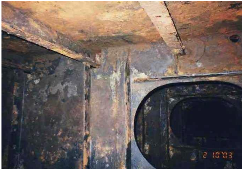
Coating Condition Sketch: POOR
