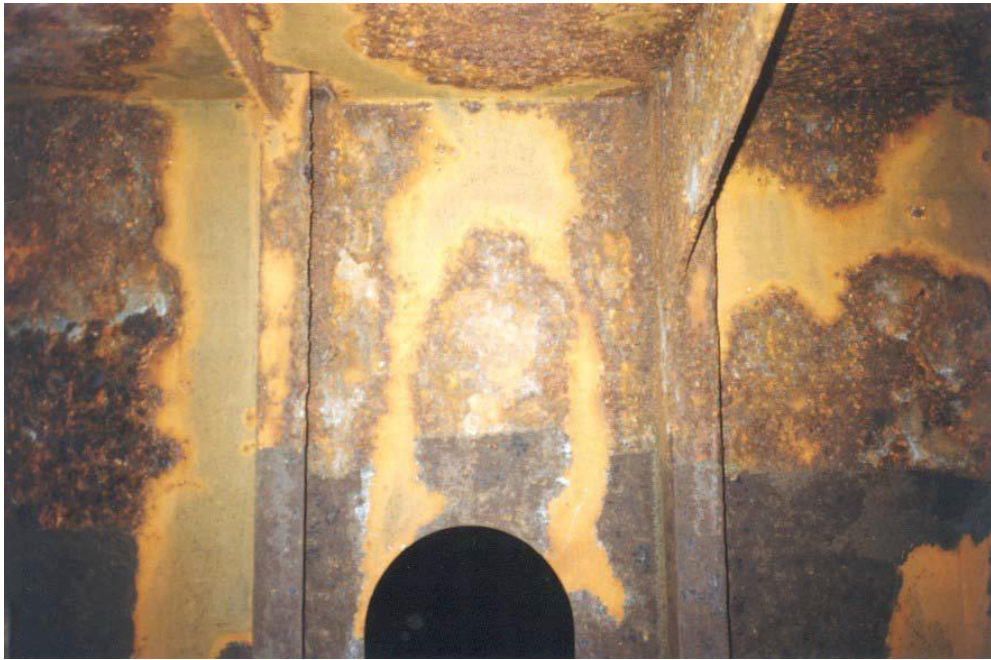
Coating Condition Sketch: POOR
