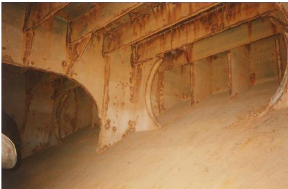
Coating condition changing from FAIR to POOR but still remaining in FAIR
